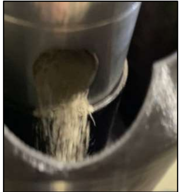
Fig. 8. Spoil is uplifted from the cutting face, through the downhole module, and into the shuttle-bucket.
