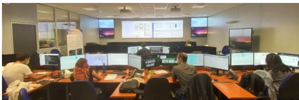
Picture 22: ROCC Main Control Room during SVT
